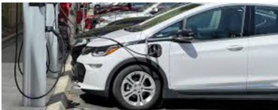
Provide Preferential parking space locations for electric vehicles
